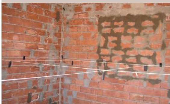
Dosimeters installed in the sealed room under construction.
