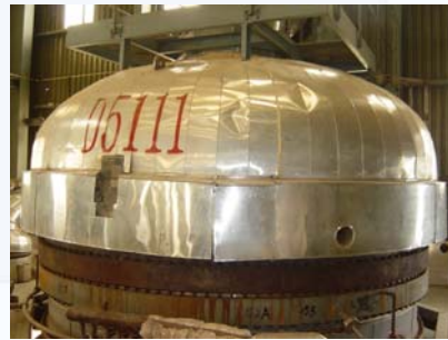
N 2 O Reactor
