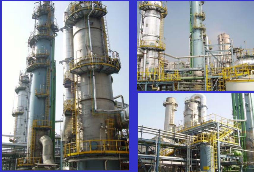
Different Views of CDR Plant
