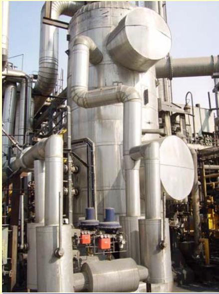
Ammonia Wash Unit
