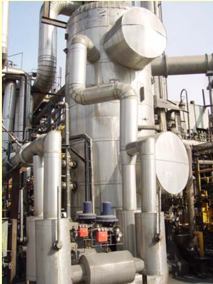
Ammonia Wash Unit
