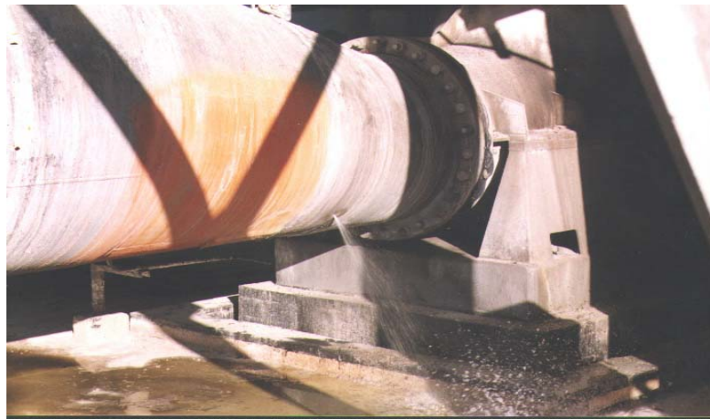
Photo-5. Phosphoric Acid Circulating Axial Pump Discharge Duct.
