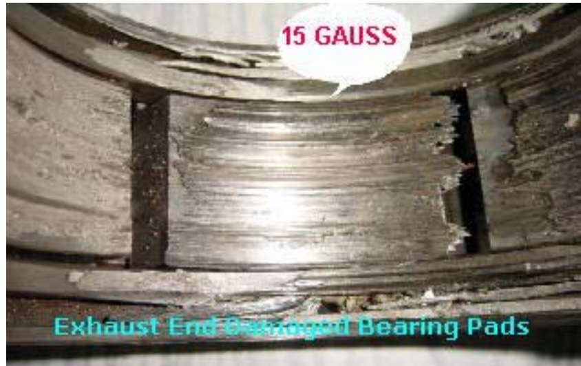
Photograph 2 Damaged Bearing Pads
