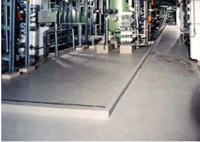
Secondary Containment with Epoxy Resin Floor
