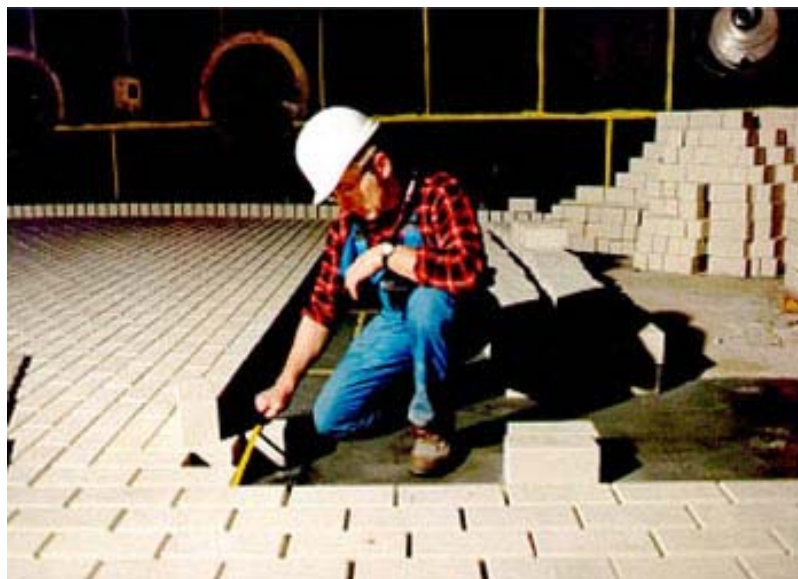
Rubber lined tank with brick protection
