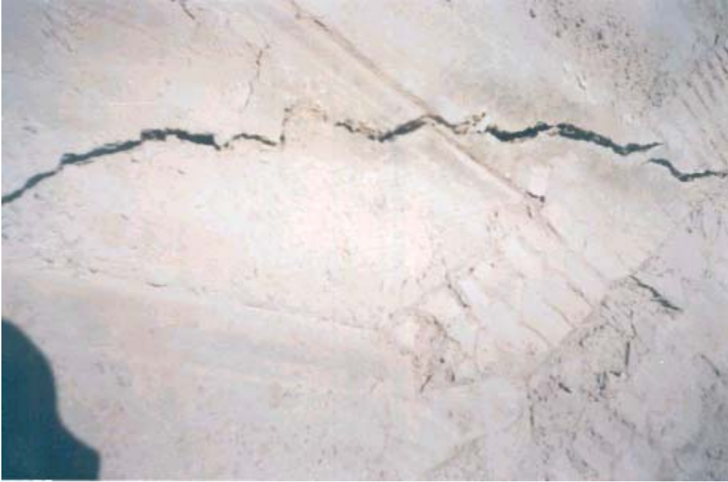
Long crack near the edge of the stack
