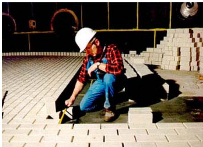
Rubber lined tank with brick protection
