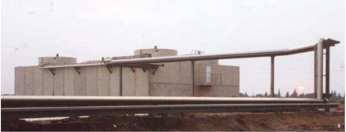
Four EMC modules for salts solution. 75000 m 3 py. Inquevap, Huesca (Spain)
