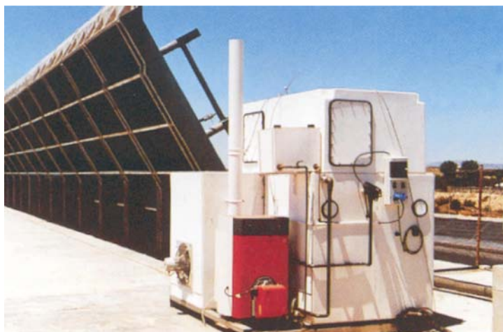
Incro's evaporation-condensation pilot plant
