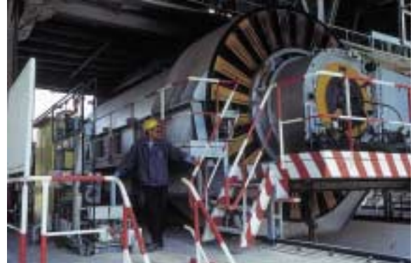
Drying plant - Office Chérifien des Phosphates (OCP), Khouribga, Morocco
