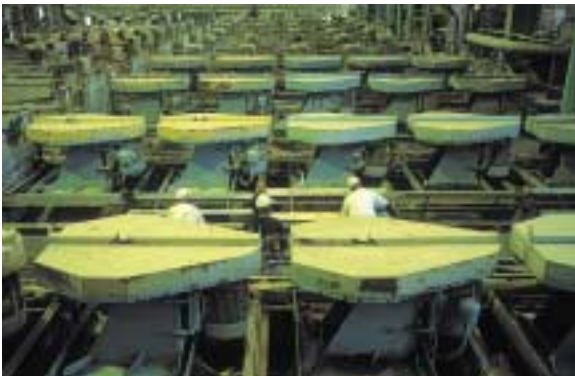
Flotation tanks - IMC Phosphate, Florida
