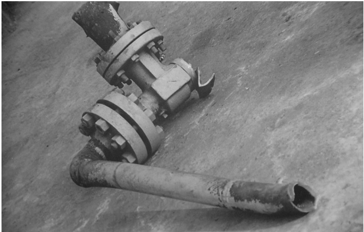
PHOTOGRAPH N°4 : RV-156-C SHEARED OFF FROM MAIN PIPE AND THROWN AWAY
