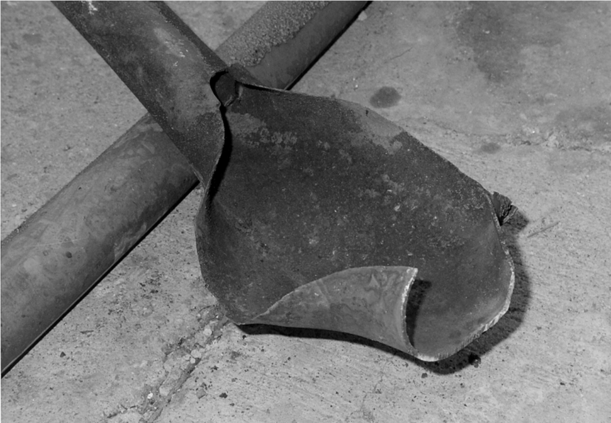
PHOTOGRAPH N° 3 : ONE TUBE IN RADIANT SECTION OF 103-B FOUND BURST OPEN
