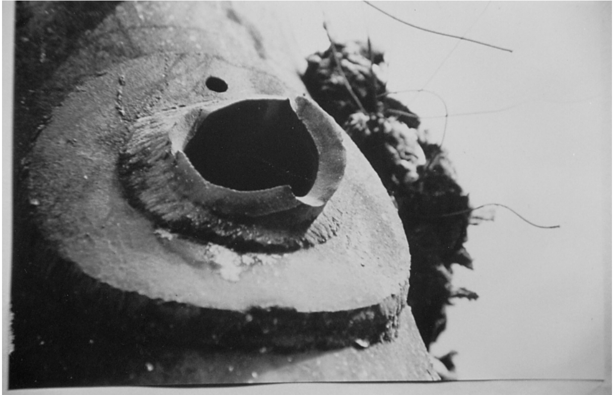
PHOTOGRAPH N°7 : RV-156-C INLET PIPE SHEARED OFF FROM MAIN 100" PIPE
