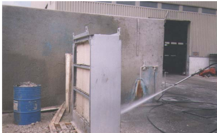
Photo-7. Gas Demister Element of Concentration Units.
