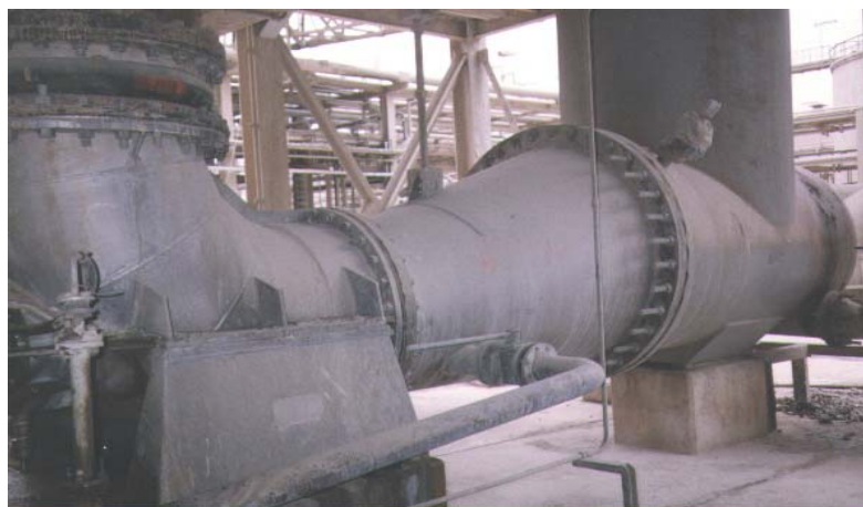
Photo-6. Phosphoric Acid Circulating Axial Pump Discharge Duct.
