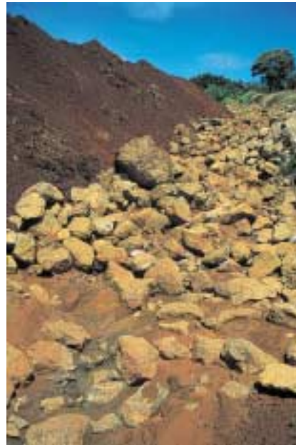
Lined drainage channel - Fosfertil, Brazil
