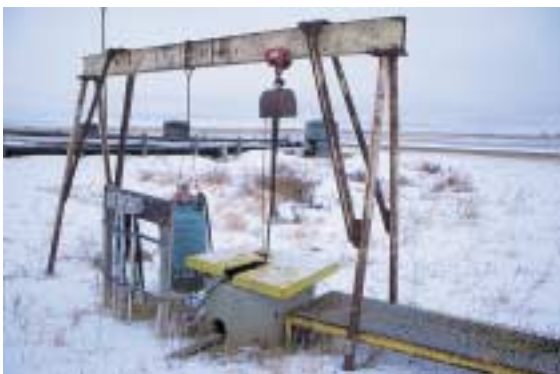
Emergency spillage recovery pump, Potash Corporation of Saskatchewan (PCS), Patience Lake, Canada
