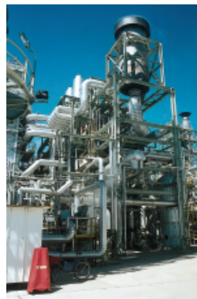
Profertil installed a silencer, a rare innovation, to prevent noise from the site bothering the local community
